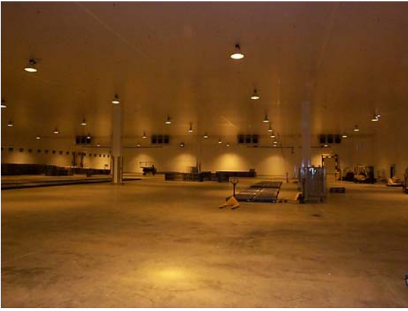
One of the three chill stores with ceiling mounted draw-through air coolers
