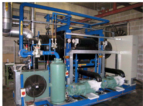
Star built Duplex Compressor / LPR packaged unit with reverse cycle defrost
