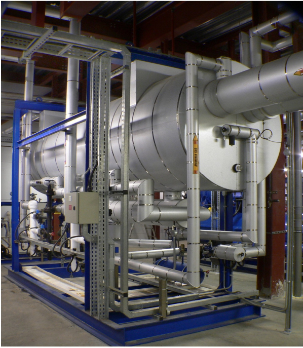
Star Refrigeration's low pressure receiver part of the central ammonia/glycol plant adopted at four Tesco distribution centres. The environmentally conscious system provides cooling for cold and chill stores and forms part of a phase out of HCFC refrigerants.
