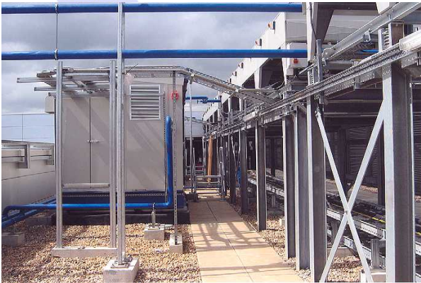
Star Refrigeration Ammonia Chillers
