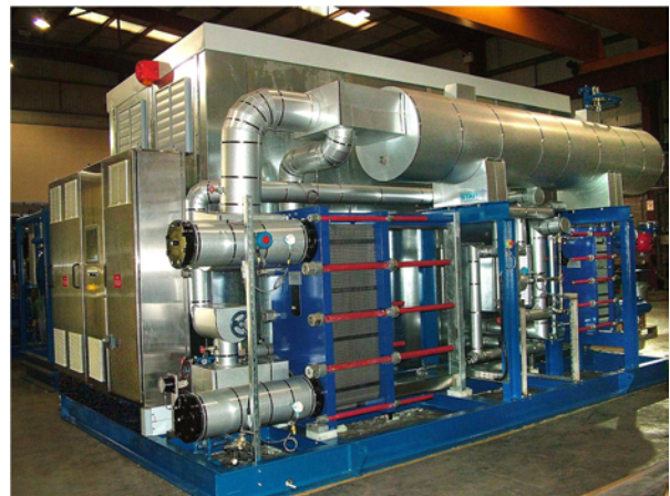
Star's low temperature ammonia water cooled chiller
