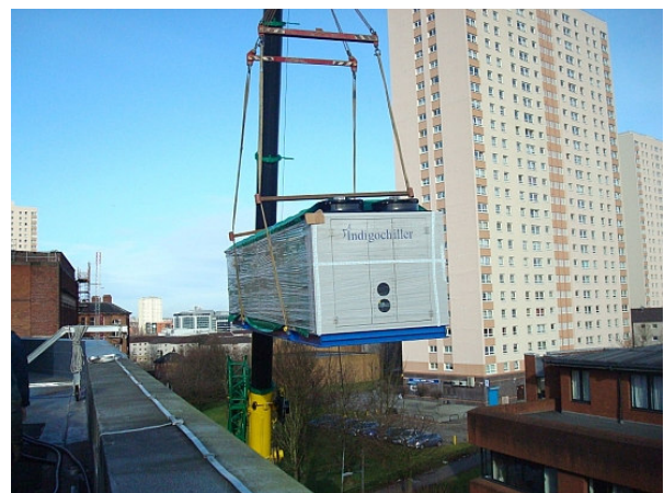
A crane lifting one of Star's Indigochillers into position on the roof of the Curran Building at the University of Strathclyde.
