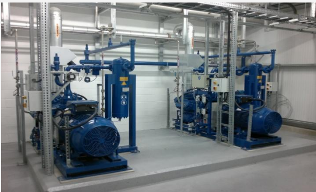
Compressor plant room
