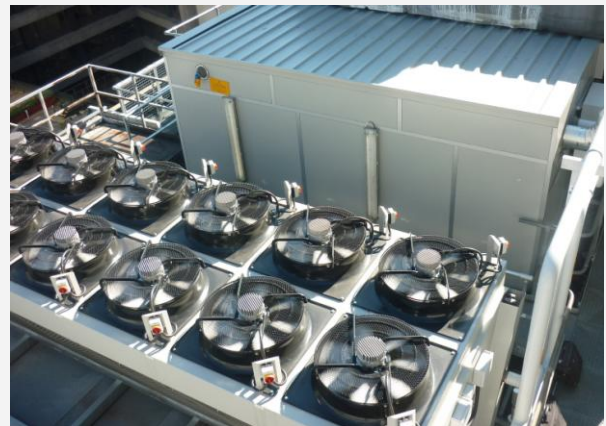
Located on the roof of the building, part of Star's bespoke high efficiency air-cooled refrigeration plant.
