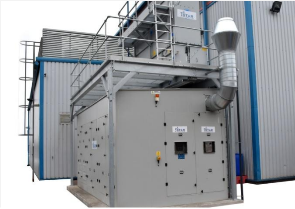
The new ammonia Glacier plant at Blakemans
