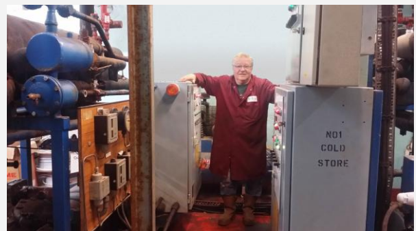
Roddy McDonald in the plant room at Associated Seafoods
