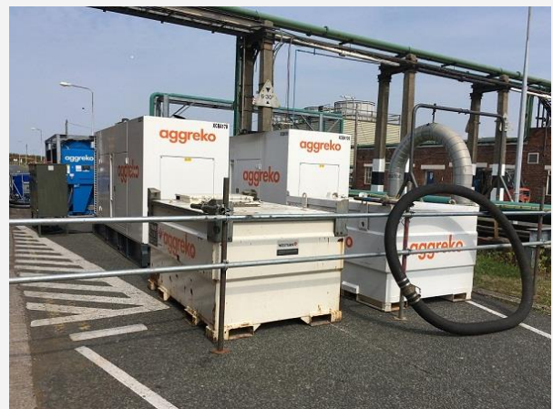
Aggreko's temporary VLTC chillers on site
