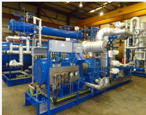
The refrigeration plant stays in line with Huntsman’s sustainability strategy by utilising zero GWP refrigerant ammonia, which will help to reduce carbon footprint.
