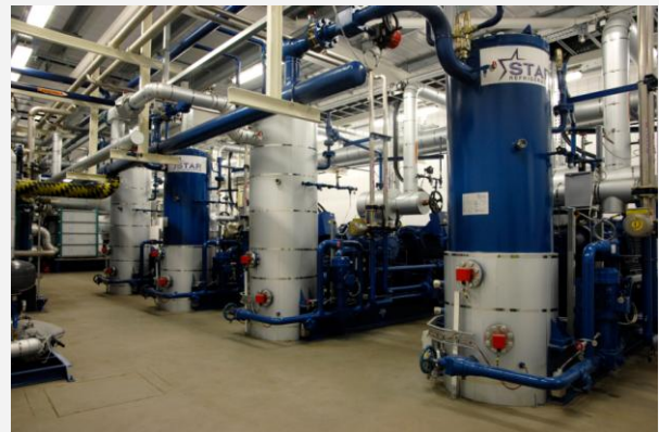
Star Refrigeration’s Neatpump at Nestle Halifax
