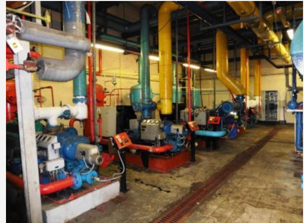
Ethos sensor panel can be retro-fitted to any refrigeration plant
