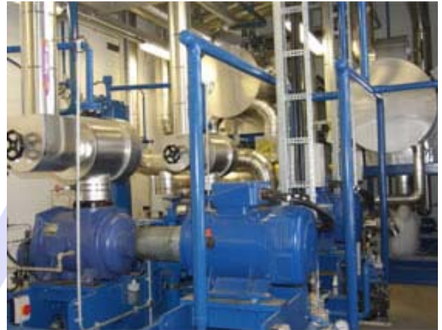
Star's energy efficient refrigeration plant which provides cooling at Macrae Edinburgh's brand new seafood processing facility. Pictured are two Howden screw compressors and ammonia surge vessels.
