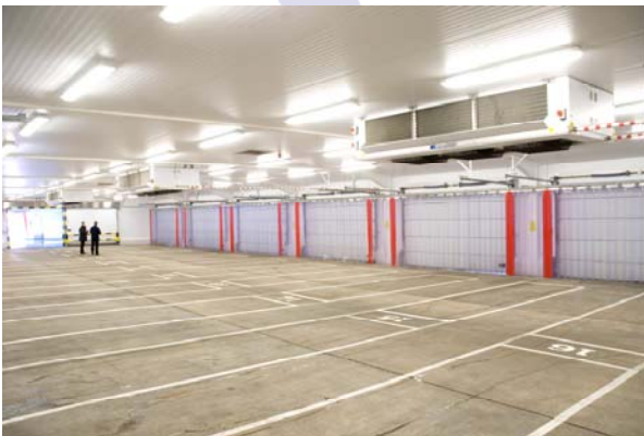
Ceiling mounted evaporator units in Harbour warehouse
