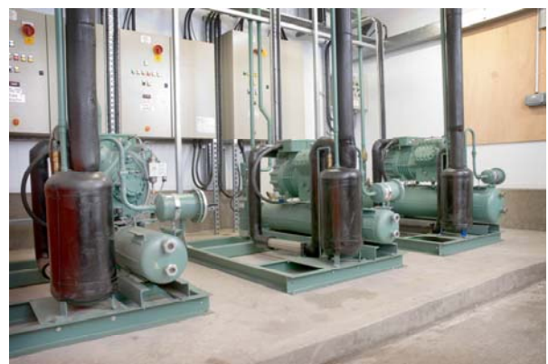
Bitzer compressor receiver units
