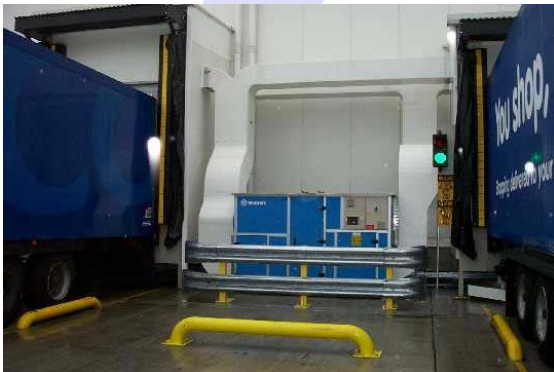
Dehumidification Unit and Ductwork
