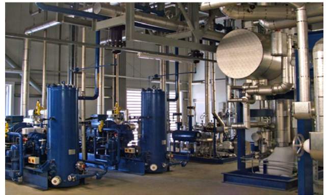
Star's energy efficient ammonia and carbon dioxide (CO 2 ) cascade refrigeration plant, installed at ASDA's Distribution Centre in Lutterworth.
