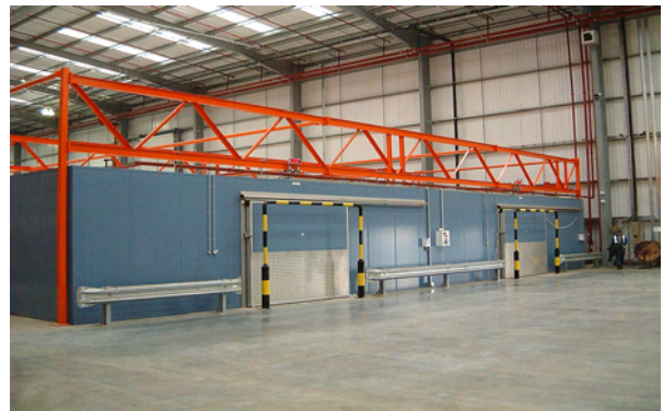
The new cold store facilities at Nisa-Today's
