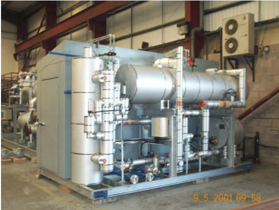
Single Howden screw compressor with drive motor and acoustic enclosure, surge drum and Vahterus plate and shell evaporator
