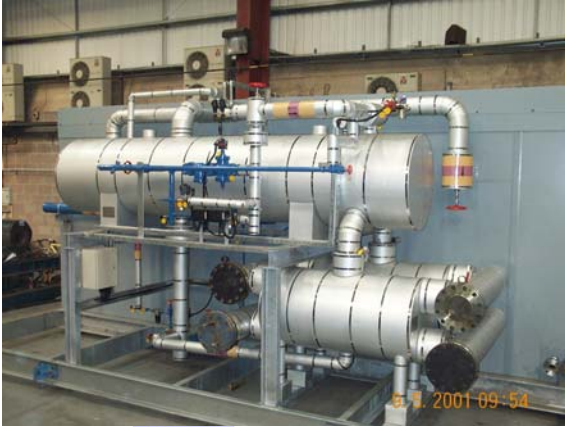
Star's custom built package including two Howden screw compressors, drive motors with acoustic enclosure, surge drum and two Vahterus plate and shell evaporators.
