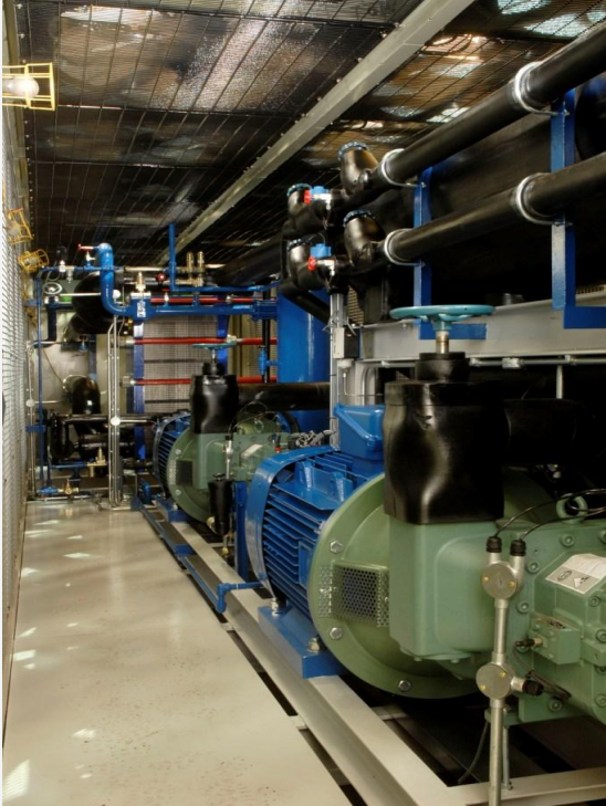
Inside the Azanechiller showing ease of maintenance
