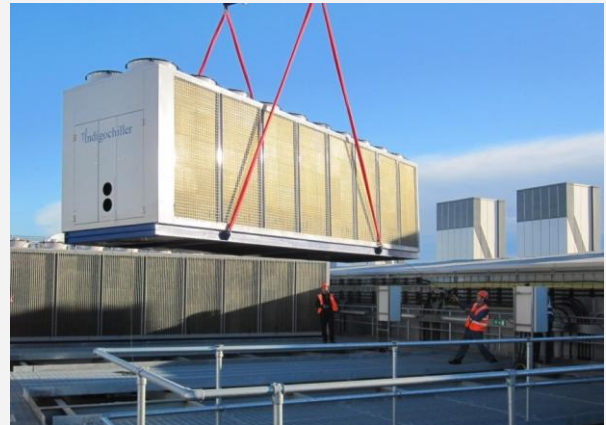
One of Star's Indigochillers being lowered onto the roof of the new Sky Studios building
