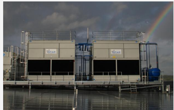
Star's high efficiency cooling system at Arla, Stourton
