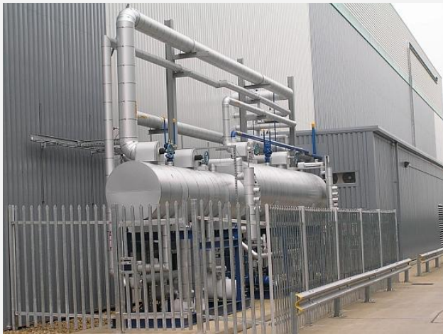
Star Refrigeration's LT & HT surge drum packages
