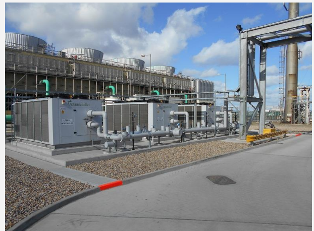
Star's air-cooled Azanechillers on site
