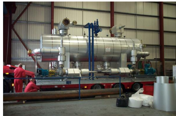
Complete tank/pump skid with latent heat storage tank, Therminol expansion tank and process pumps
