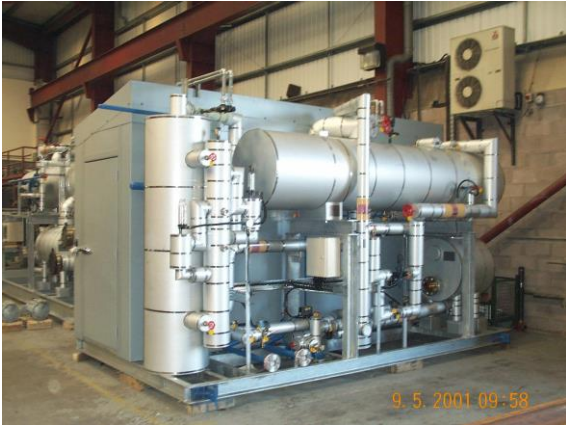
Single Howden screw compressor with drive motor and acoustic enclosure, surge drum and Vahterus plate and shell evaporator
