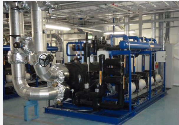
Inside the plant room - Star's high efficiency chiller package for data centre cooling
