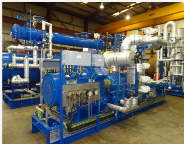
The refrigeration plant stays in line with Huntsman’s sustainability strategy by utilising zero GWP refrigerant ammonia, which will help to reduce carbon footprint.
