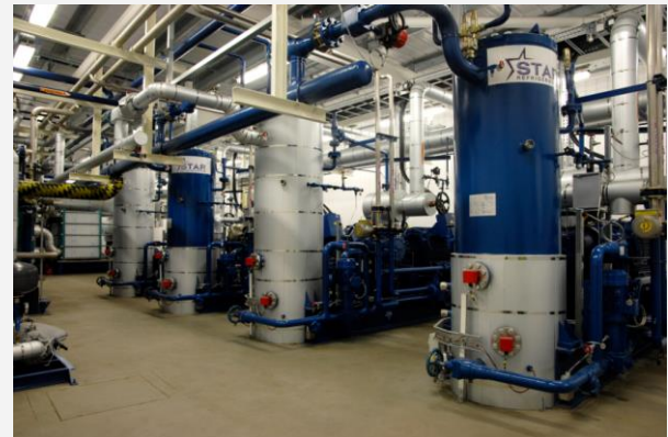
Star Refrigeration's Neatpump at Nestle Halifax
