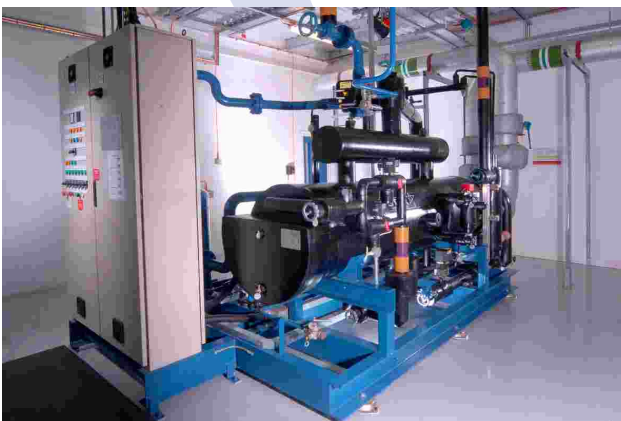
Freechiller plantroom packaged unit
