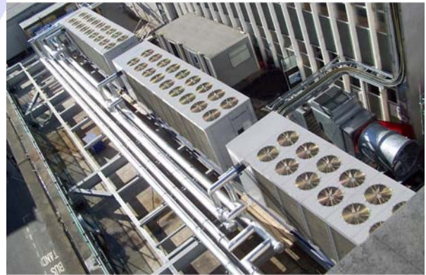
Three of Star’s Indigochillers on the sixth floor roof of the John Lewis department store in Oxford Street, London
