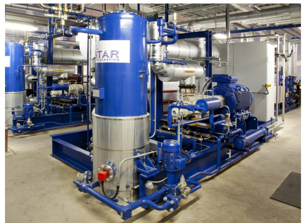
Star's multi-temperature cooling system for Brakes comprises four LPR (low pressure receiver)
