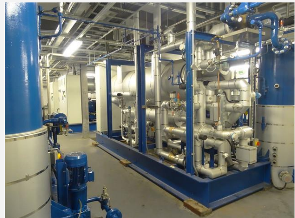
Ethos connected to refrigeration system
