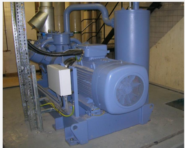
The new compressor package installed by Star Refrigeration
