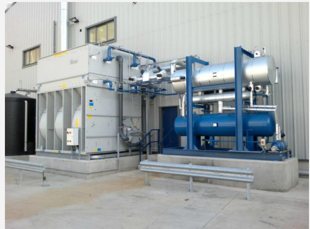
Evaporative condenser connected to the combined surge drum and high pressure receiver package unit
