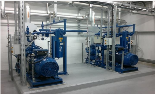
Compressor plant room
