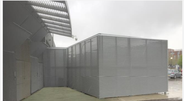
New Azanechillers in location
