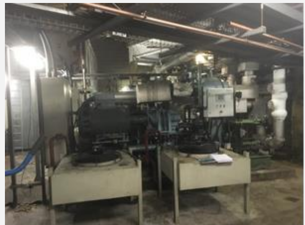
Existing plantroom R404A chillers
