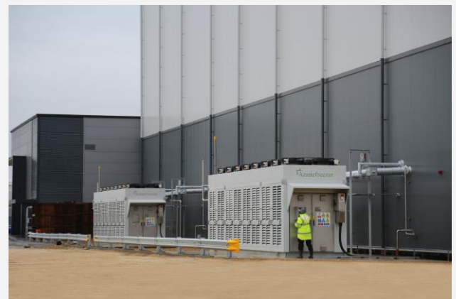
Azanefreezer installed at Lineage Logistics, Great Haddon
